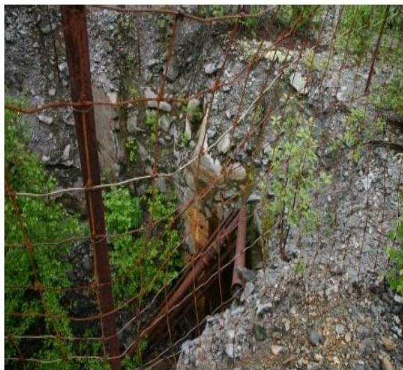
Plate 1. Caved shaft collar at Norpax deposit
